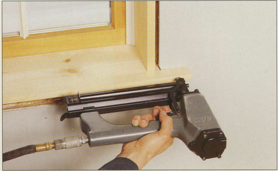
A window sill, or stool, is fastened to the wall studs with a finish nailer. Cut to fit the window opening, the stool features horns that extend past the window frame.
