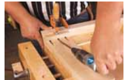
Be sure to glue the joint and hold the leg and apron together tightly while screwing it together.
