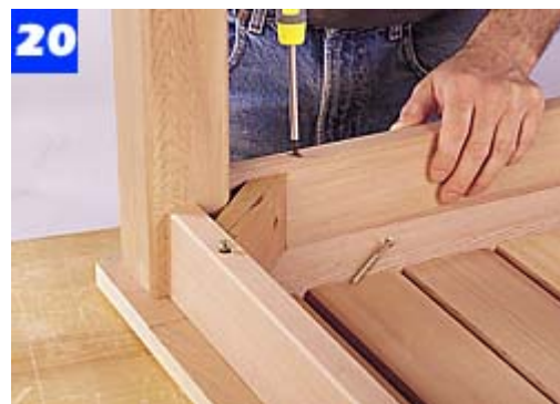
Attach the tabletop to the base with several screws. Drive each screw into its matching counterbored hole in the apron.
