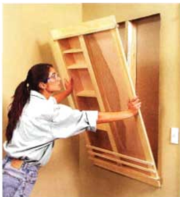
10 Set the completed message center in the opening and level it. Then nail through the trim into the studs to secure it.
