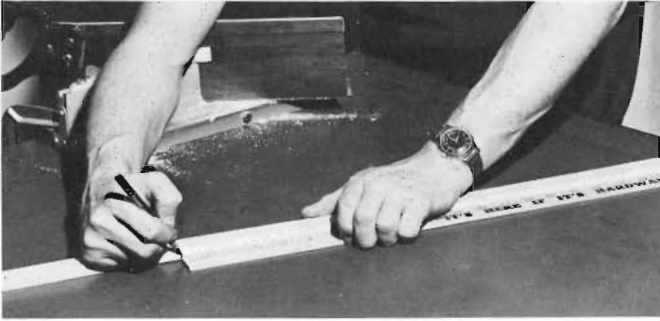
7 Measuring. Mitered pieces will normally be measured on the inside or short edge of the molding. However, when we assemble the insert, the square edge of the molded stop has to match the outside edge of the rabbet strip; therefore we are measuring 21\frac{5}{8} inches (54.9 cm) along the outside edge.
