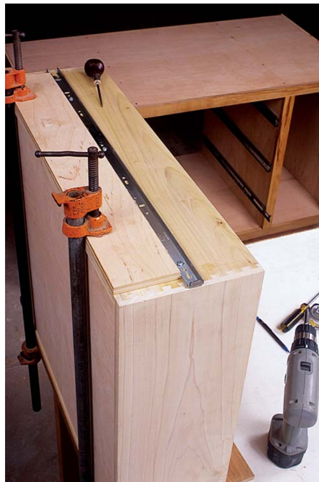
PHOTO I: After centering one drawer-half of a slide on a drawer, make a spacer for installing the slides on all of the drawers.
