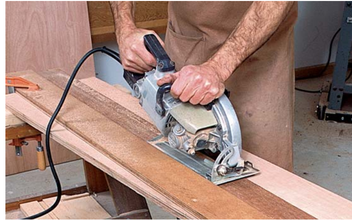
PHOTO C: Saw the angled braces with a portable circular saw guided by a plywood straight edge.
