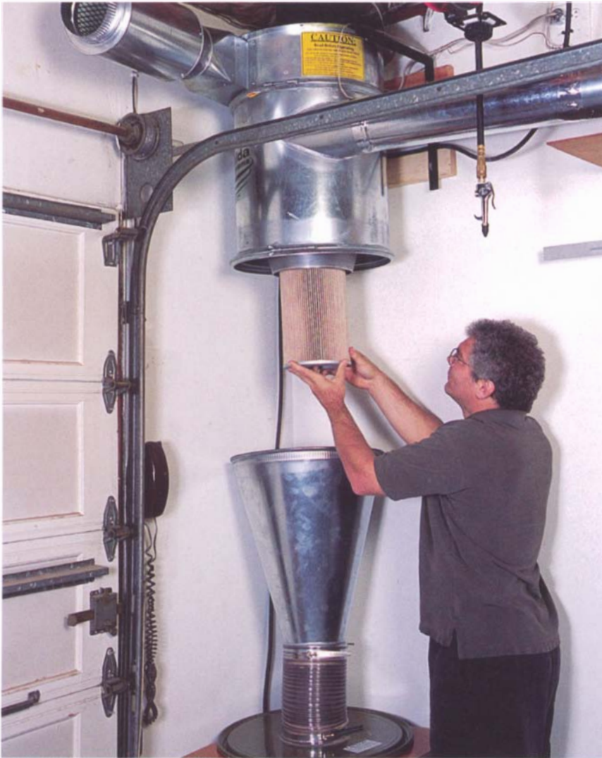
A cartridge filter made for central dust collection is much like a pleated filter used in a shop vacuum. Here, woodworker Matt Bays replaces the filter in his Oneida cyclone/blower, which uses the cartridge in lieu of filter bags.
