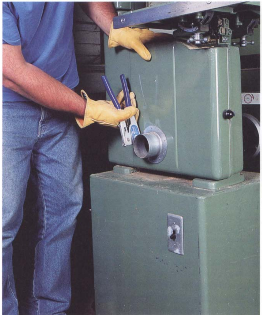
An angle-ring fitting pop-riveted over a hole cut into a flat metal surface, such as the lower blade enclosure on this bandsaw, provides a dust-collection port and a sturdy attachment for a flexible hose.
