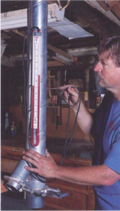
A tube-style manometer and Pitot tube can be used to check static pressure, air velocity, and air volume moving through a duct. With the Pitot tube inserted into the duct through a small hole, fluid is displaced in the manometer tube, giving a reading as inches of pressure on the scale.
