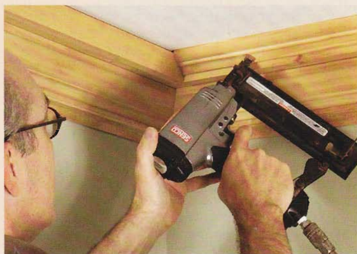
8 Install bed molding between the fascia and ceiling. If necessary, you can caulk any gaps between the molding and ceiling or wall surfaces.
