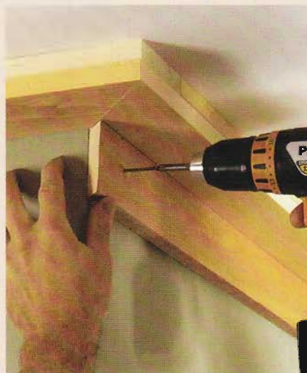
4 Mark a level line to indicate the bottom edge of the frieze. Use screws to fasten the frieze to wall studs or top plate.
