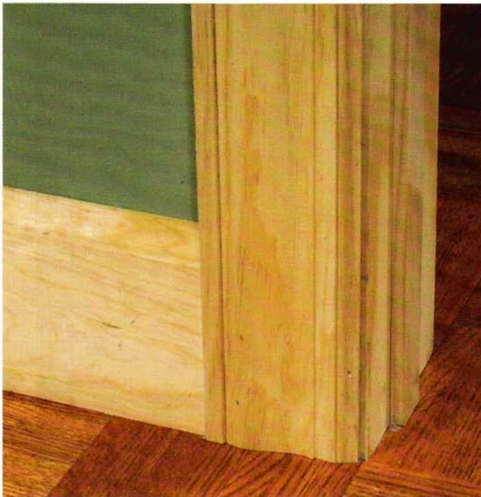
Detail of one-piece baseboard with stock Colonial door casing.
