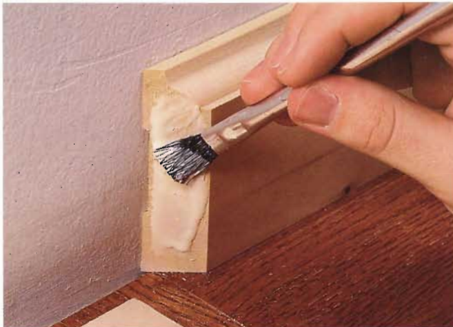
4 Apply wood glue to both sides of the joint. (You will need to wipe off some excess after nailing.)
