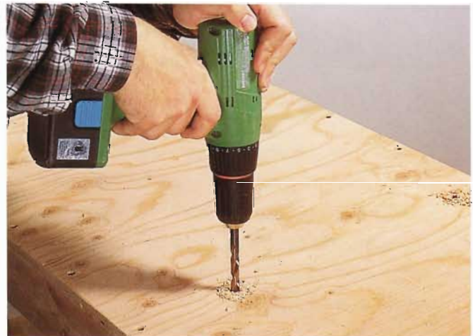
5 Drill bolt holes through the platform. If the holes fall on the 2x4 frame, you can use lag screws instead of bolts.
