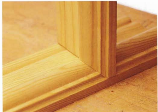
7 Test the cut on a piece of molding with the same profile, and make final adjustments as needed before fastening.
