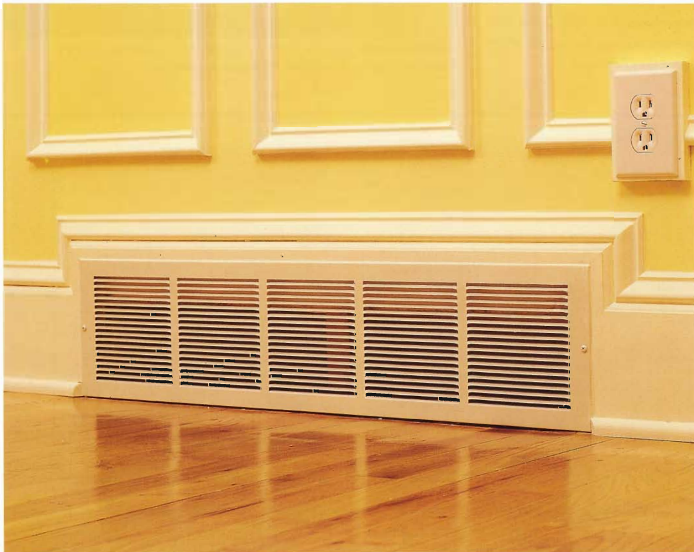
This register is neatly framed by carrying the top couple of inches of the baseboard and base cap molding around the top edges.
