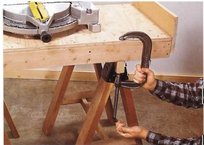
8 Set up your saw bench near the work area, clamping it firmly to stable sawhorses.
