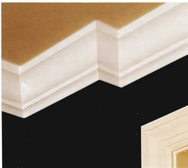
Painted cornice molding turns inside and outside corners without showing any trace of the cut joints.
