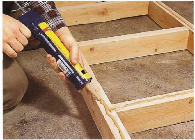
2 Increase stability of the assembly by adding construction adhesive to the top edges of the 2x4s.
