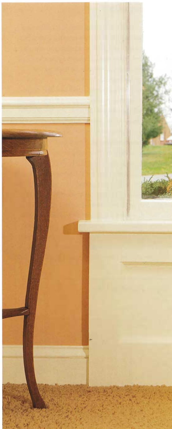
The horns of a window stool extend beyond the casing.
