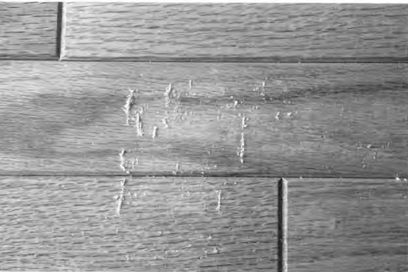
Some water-based products may not adhere to solvent-based finishes. This flooring sample was coated with rubbing oil and then sprayed with a water-based lacquer. The dry finish scraped off the surface without too much effort.
