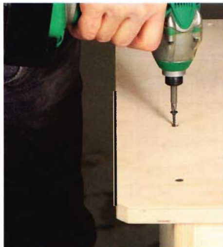
No glue needed. Drywall screws provide plenty of holding power, so there's no need to fuss with glue.
