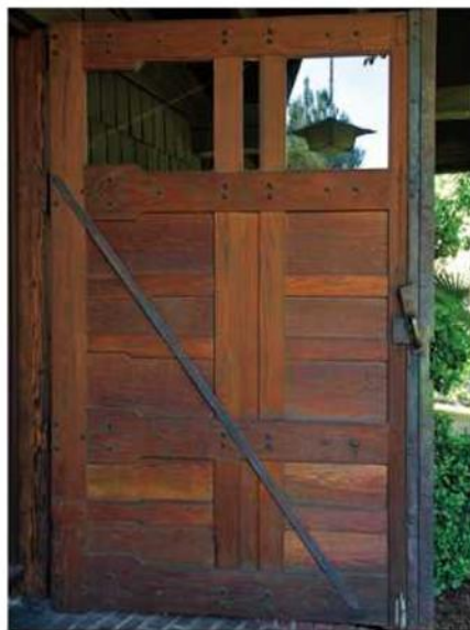
Outbuildings, not afterthoughts. The garage doors at the Gamble house contain cloudlift rails and panels, a feature that recurs throughout the main house.
