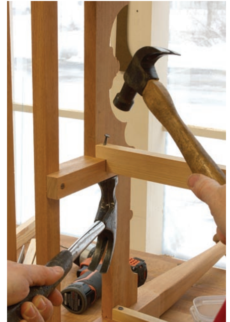
Absorb the blow. A second hammer placed directly behind the nail allows you to attach the runners to the dividers without problems.
