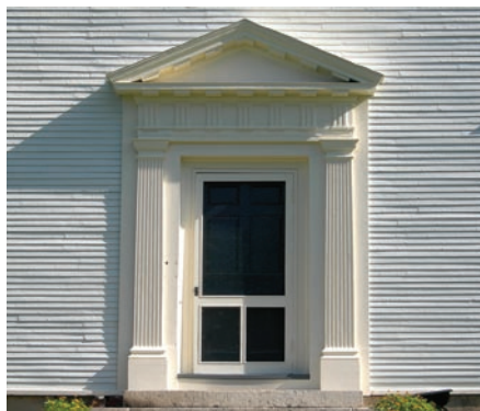
A statement. The mouldings surrounding this door make it plain to all that it is an important entry.
