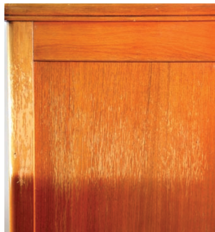
Fading finish. Notice the fading and finish deterioration in the top two-thirds of this cabinet, which backed up against a west-facing window for many years.
