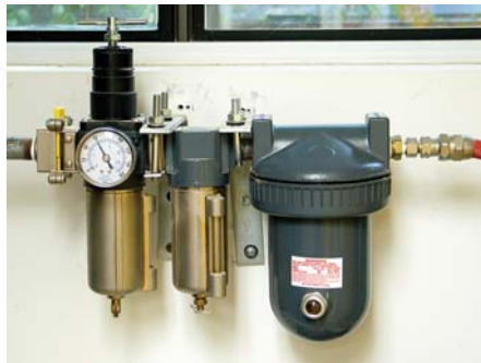
Regulator. Both methods of optimizing the air pressure to a spray gun can be done with just a regulator, which is attached to smaller, portable compressors and is mounted on the wall with larger, stationary compressors. This picture shows air and moisture filters along with the wall-mounted regulator.
