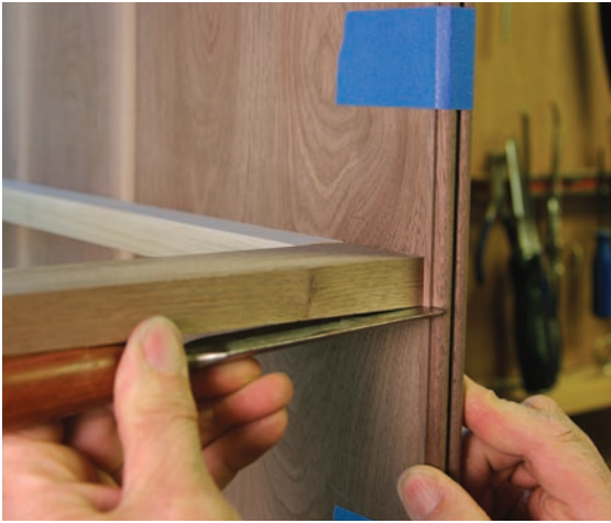
Accuracy is important. A sharp chisel marks the beaded moulding exactly at the place the V-shape is to be cut.
