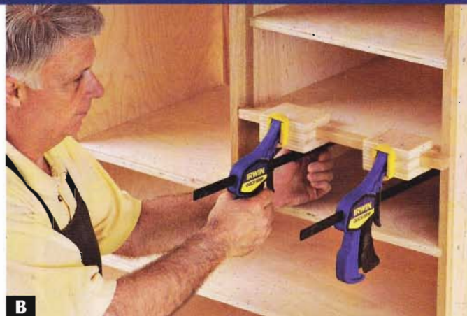
B Clamp the edge banding into place. To give the far clamp jaw a surface to bear on, apply the edge bands with the case back off.
