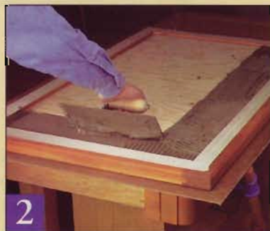
2 Protect the frame with tape, then spread the mortar with the trowel. Form ridges in the mortar with the notched edges of the trowel.
