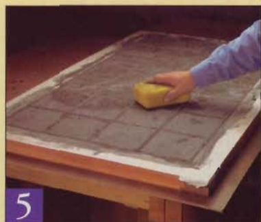
5 As the grout dries, wipe off the excess with a sponge and clean water. Repeat this many times to clear away the dried film.
