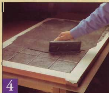
4 After the mortar sets, fill the gaps with grout. Force the grout into the gaps by pushing the float diagonally across the tile.
