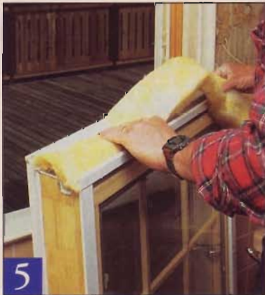
5 Before you set the new window in place, turn it upside down and tuck a layer of fiberglass insulation under the sill.
