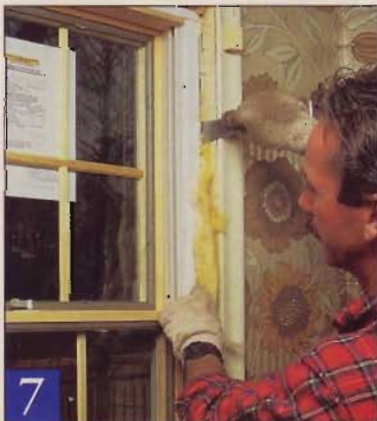
7 Once you've checked the window for square, tighten the screws, then cut the shims off and press in some insulation.
