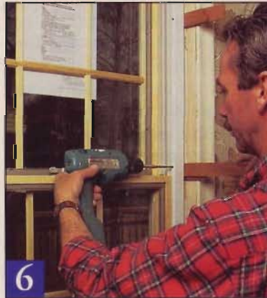
6 Place wood shims between the new window frame and the old jamb (at the screw locations), then partially drive the screws.
