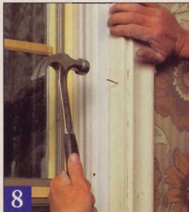
8 Nail the inside stop molding back in place. If swinging a hammer next to glass makes you nervous, use a cardboard shield.
