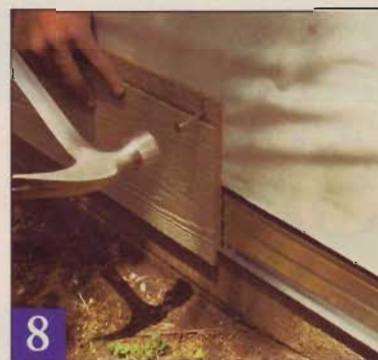
8 Begin by nesting the starter siding course in the starter strip and nailing through the top flange. Locate any joints over studs.
