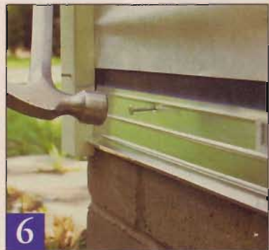
Some starter courses go directly against the wall, but LockSide requires a metal strip to hold the siding in at the base.
