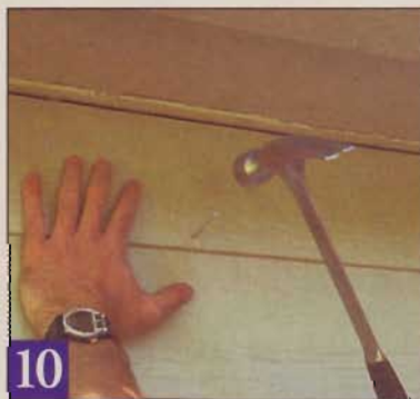
10 The last course of siding will probably have to be trimmed to fit, removing the top flange. Face-nail these pieces.
