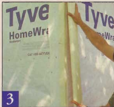
When making battens for outside corners, be sure to rip one batten narrower than the other to keep the assemblies symmetrical.
