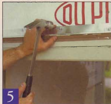
Aluminum flashing above header trim will divert water away from the tops of windows and doorways, keeping them dry.
