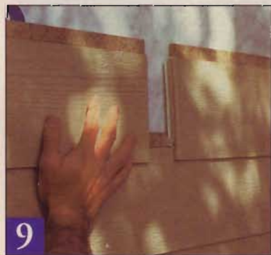
9 Custom-matched aluminum joint moldings help seal splices on long walls, but caulk will add some extra insurance.
