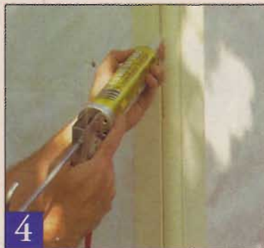
A decorative edge dresses up this batten corner, which is caulked at the wood joint and where each board meets the wall.
