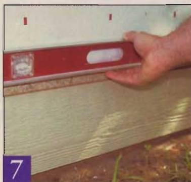
7 With the metal starter strip tentatively nailed in place, hang a length of siding and check it for level and baseline height.
