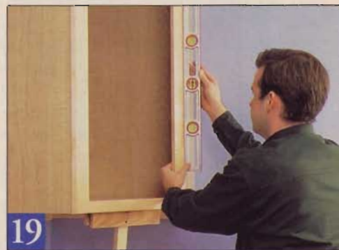
19 Set the corner wall cabinet on the ledgers and, if necessary, shim it until the frame is plumb. A T-brace supports the front.
