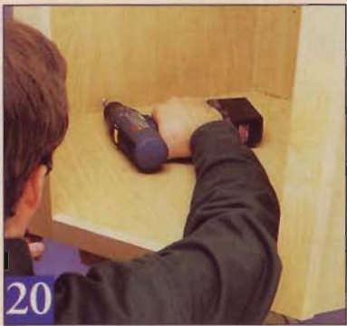
20 Drive mounting screws through both the upper and lower hang rails in each upper cabinet. Aim for a stud on each wall.
