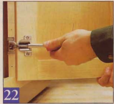
22 When the last cabinet has been secured, you can replace the doors, drawers, and shelves. These hinges provide adjustment.
