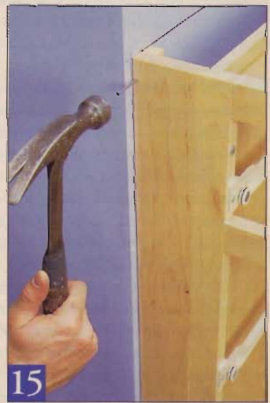
Drive screws from the end face frame into the edge of the filler board, then nail the other side to the support cleat.
