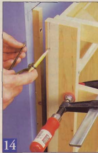
If the end wall is irregular, scribe-fit the filler board. Plumb it against the end unit, trace the contour, then cut on the line.
