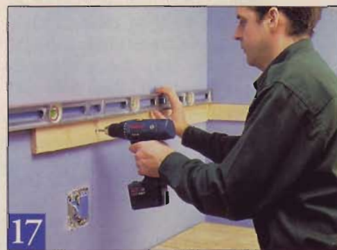
17 Ledger boards, set at the upper level line, provide temporary support for the upper cabinets. Make sure the screws hit studs.
