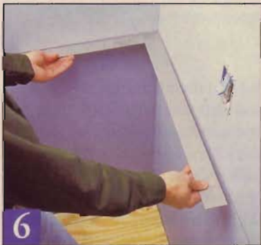
6 An out-of-square corner might require you to adjust the location of the toe kick baseline on the floor, so check each one.
