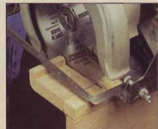
To cut a post-formed countertop, begin by sawing through the backsplash with a fine-toothed blade.
