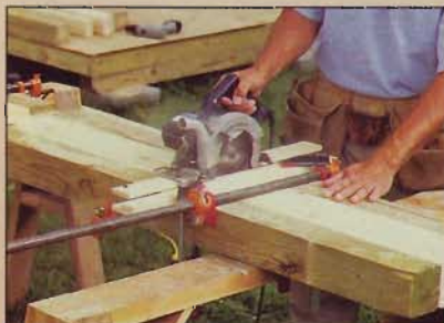
Align and clamp together the studs and posts for one wall frame. Mark layout lines for the notches, then make a series of 3/4"-deep cuts.
