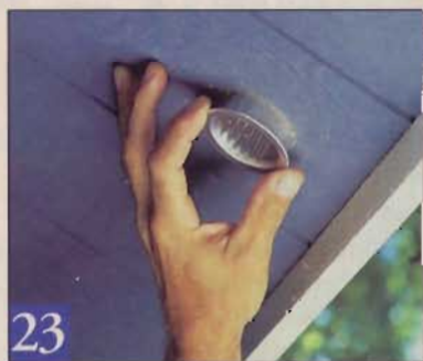
23 We used self-rimming soffit vents, fitted with screen mesh that keeps out insects. They press in, so the fit has to be snug.
