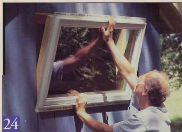
24 After we painted the siding, we installed our awning window in the rear wall. The nailing flange will be covered with trim later.
