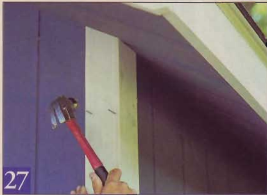
27 Cedar battens butt together to trim the corners. Install the narrow battens on the side walls, the wide trim on the ends.
