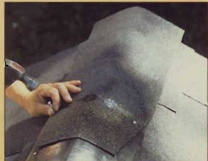
After nailing on a ridge vent, cut some "three-tabs" into 12"-square shingles for the ridge. Install with a 5" reveal, same as on the slope.
