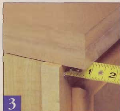
3 The edge of the substrate must be parallel to the face of the base cabinets to ensure a uniform overhang.
