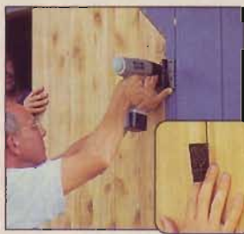
Use a shim (or an extra hinge plate) to create a 1/8" gap around each door edge.
