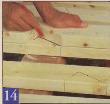
14 Test fit one or two rafters to get the dimensions right, then use the "pattern" rafter to do layout marking on the rest.
