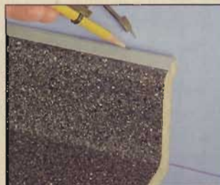
After aligning the front edge with the cabinets, scribe the backsplash to the wall with a compass.
