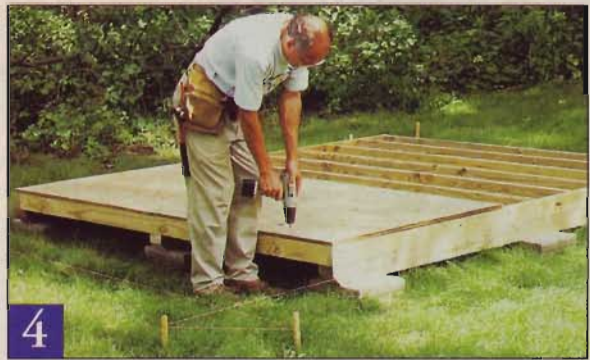
Align the frame and skids, check for square, and fasten them together. Then screw the plywood flooring to the joist platform.
