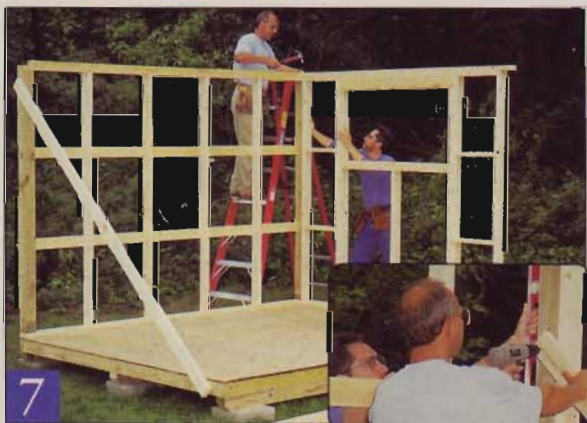
With one side wall screwed to the floor and held by a temporary brace, set and plumb the rear wall, then nail the plate corners.
