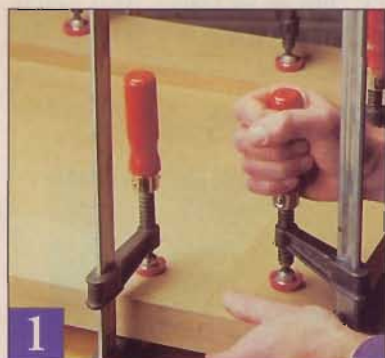
1 Build up the substrate edge thickness by gluing 4"-wide cleats of Medex to the bottom sides of the countertop substrate.
