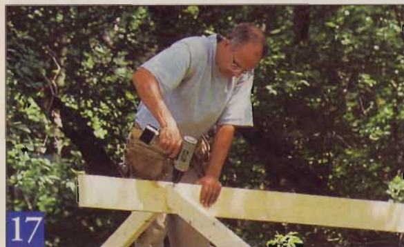
17 The loft makes a nice work platform for installing the ridge beam. The beam's front end overhangs the shed by 18", the back by 6".
