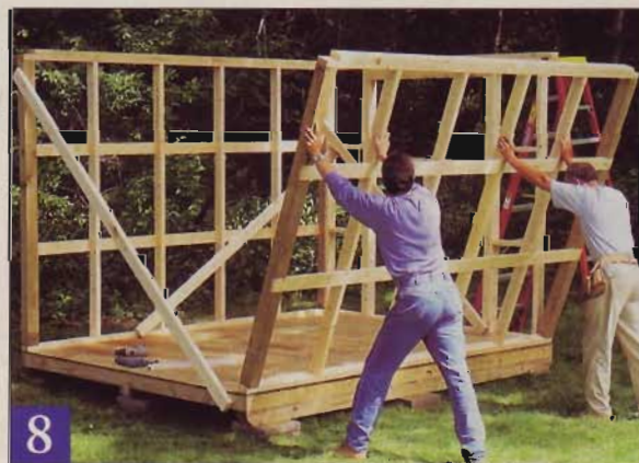
Work your way around the shed perimeter as you raise the walls. Most of the braces should stay until after the siding goes up.
