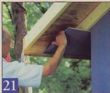
21 The angled groove cut in the fascia boards provides support for the soffit panels. The top edges rest snugly against the siding.
