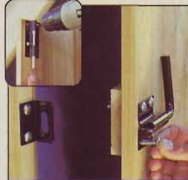
The left-hand door gets slide bolts top and bottom (inset); the right door gets the latch.
