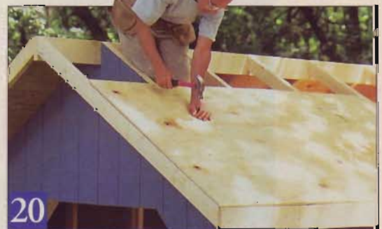
20 You can nail the sheathing down as soon as the roof frame is complete. Start at the bottom edge, and offset the end joints of the lower and upper panels as you work up.
