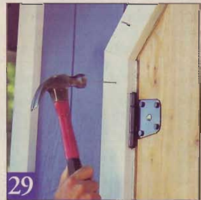
29 The routed pockets nest over the hinges. Cut the ends of each trim piece at 22 1/2° to turn the 45° corners around the door.
