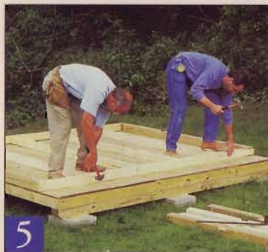
5 Use the shed floor for a work platform as you build the walls. The notched edges of the studs and posts should face up.
