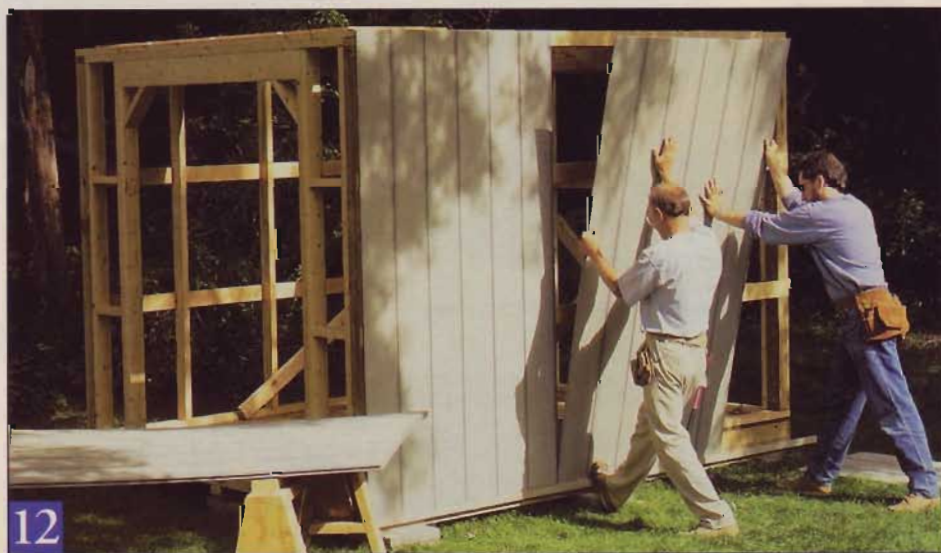
12 A temporary ledger board provided support for the siding panels while we installed them. The bottom edge of the siding extends \frac{3}{4} " below the top edge of the skids.
