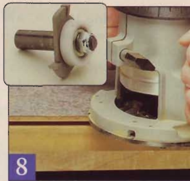
8 Using the slot cutting bit sold by the edging manufacturer, rout the edging mounting groove in the edge of the substrate.
