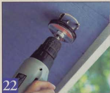
22 Drill 2" holes in the soffit panels (between the rafters) to house the soffit vents. Test fit a vent in scrap before drilling the holes.
