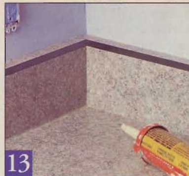
Install the longest piece of backsplash first, then install the coped piece against it. A bead of caulk wraps it up.
