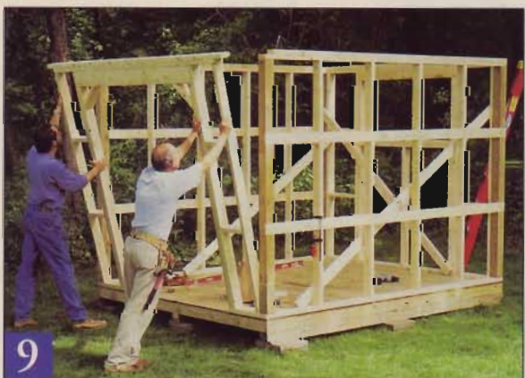
We fastened the top plate to the front wall before raising it, then nailed the extended ends to the wall plates of the side walls.
