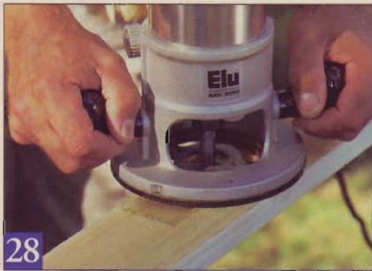
28 Mark the hinge locations on the inside face of the door trim and trace around a hinge plate. Then rout a shallow mortise.
