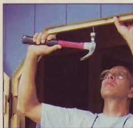
We nailed cedar 1x2 stock in place for a door stop molding. It also helps keep insects out.
