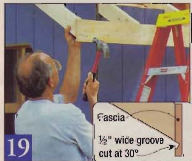
19 Cut an angled groove (for the soffit panels) in the fascia, then nail it to the rafter tails. The fly rafters can then be nailed in place.
