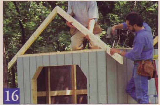
16 Install the first rafters at the ends of the shed, fastening them to the top plates. The center gap at the top measures 1 1/2", enough room to accommodate our 2x6 ridge beam.
