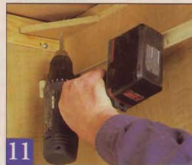
11 Before you remove the bracing, drill pilot holes through the cabinet corner braces, and drive screws into the substrate cleats.
