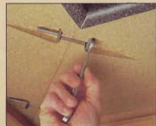
After applying a bead of silicone caulk, use drawbolts to pull the countertop joint tightly together.
