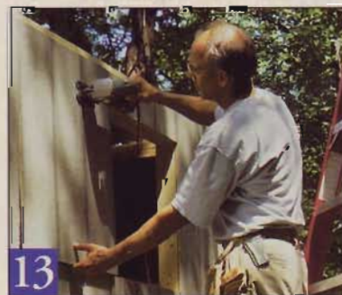
13 Mark the window corners by drilling small guide holes from inside the shed, then lay out and jigsaw the cutout in the siding.
