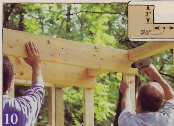
Notch the loft beams so the top edges are flush with the walls. Set two beams for the rear loft, skip a stud, then add front beam.
