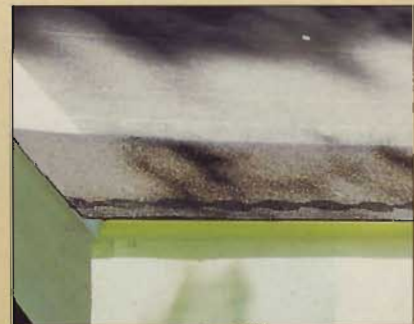
A starter course makes for a double layer of shingles at the bottom edge of the roof. Cut the tabs off regular shingles to make these.
