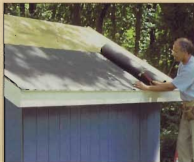
Builder's felt is the first layer of protection for the sheathing. Cover the drip edge and work up. Add rake flashing at the ends.
