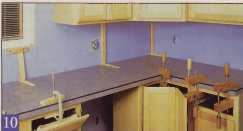
10 Install braces against the upper cabinets near the back edge and clamps along the front. These hold the countertop firmly in position until the construction adhesive dries.
