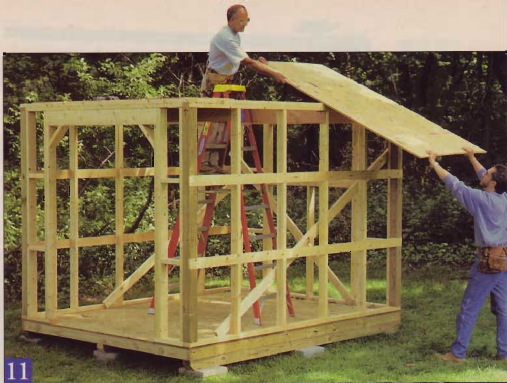
11 The loft plywood has to go on before you get to the roof framing. We cut our panels 86" long, notched the outboard edges for the ridge posts, then screwed them in place.
