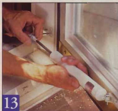
13 Drill pilot holes and mount the brackets to the door and jamb. Install the closer and adjust its closing tension.
