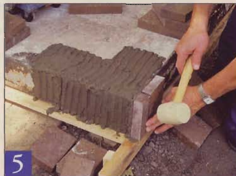
5 Trowel mortar onto the corner of the slab, covering just the area where you'll set the first corner pavers. Set the riser pavers first with taps from a rubber mallet.
