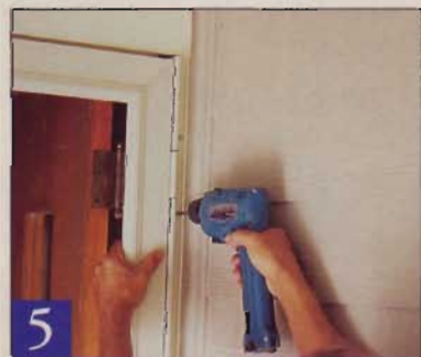
5 When the hinge jamb is plumb, install the top front-facing screw. Re-check your level before driving the rest of the screws.
