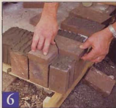
6 Spread mortar on the top end of each riser, stopping about 3/8" from the front faces. Then set the corner pavers in place.
