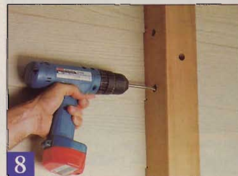
8 Drill 5/8" holes through the posts. When the tip of the spade bit protrudes, finish drilling from the opposite side. Eyeball your alignment so the bit stays on course.
