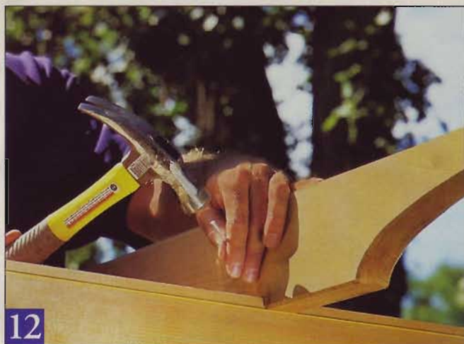
12 Toenail the rafters to the beams, driving two galvanized casement nails at each rafter notch location (see the Pro Tip below). To prevent racking put one nail in from the left side of the rafter and one from the right.
