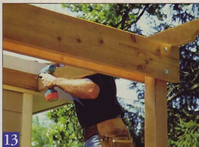
13 Once the outermost rafter was in place, I cut the ledger to length. With some help, I screwed the ledger to the fascia, locating the screws so they would be covered by the ends of the rafters.
