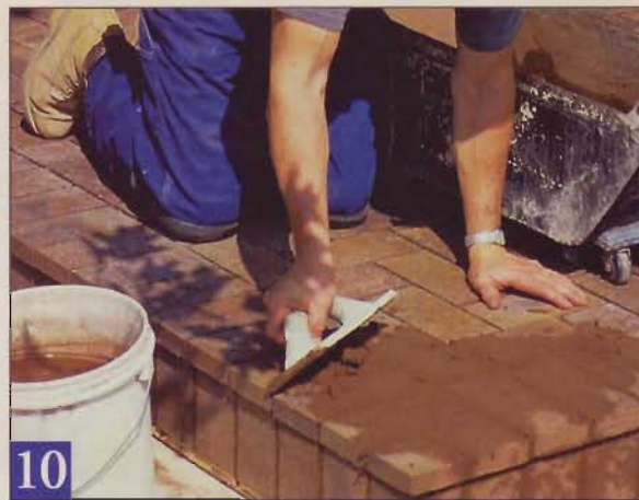
10 Work grout between the pavers with a float. Then tilt the float to 45° and scrape diagonally across the pavers to remove the excess.
