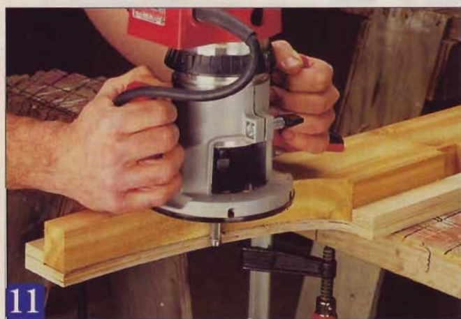
11 Clamp the rafter tail template in place and rout the rafter blank to shape with a flush-trim bit. Cleats on the template prevent the stock from shifting.
