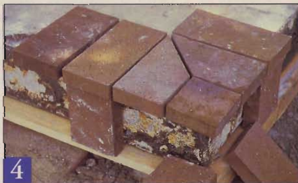
4 Miter two pavers at 45^\circ and cut another one in half to fill the corner. Set the risers on the ledger board so they align with the soldier course pavers. You'll have to rip the risers that meet at the corner.
