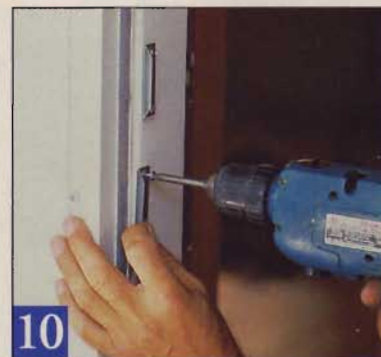
10 Close the door to align the striker plates for the latch and deadbolt. Mark the jamb, then you can open the door to install them.
