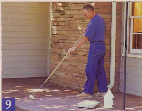
9 Lyle applies a coat of exterior masonry sealer to the pavers before grouting. This prevents stains caused by grout and water.
