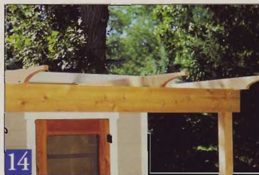
14 Installing intermediate rafters establishes uniform distance between the beam assembly and ledger. The stringline along the top edge of the outer beam provides alignment.
