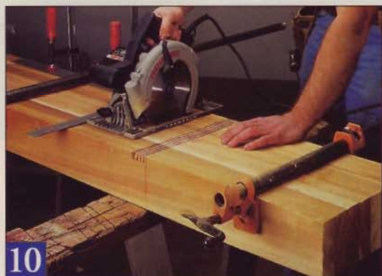
10 Clamp the rafters together and gang-cut the notches with several passes of a circular saw. Chisel out the waste.
