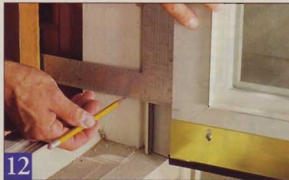
12 Mark the position of the closer mounting bracket on the interior face of the door. Then use a square to transfer the bracket alignment to the side face of the door jamb.
