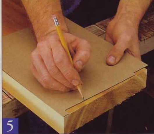
5 Scribe the siding profile onto an 8"-wide piece of cardboard. Cut this template to shape and use it to transfer the siding profile onto the end of each beam.
