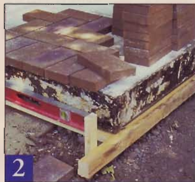
2 Ledger boards position the riser bricks flush with the porch surface, and hold them in place while the mortar sets.
