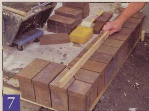
7 Working each way from the corner, set the riser and soldier pavers. Watch the chalk lines to keep things square, and check the surface with a straightedge.
