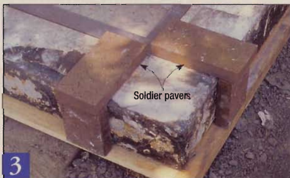
3 Align a framing square with the chalk layout lines and position the first two pavers in the soldier course. Set the pavers against the square, but offset each \frac{3}{8} " from its corner to leave space for grout.
