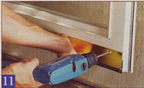
11 Carefully slide the sweep onto the bottom of the door to prevent scratching the finish. Adjust the sweep to fit snugly against the sill, then drill pilot holes and drive screws to hold the sweep place.
