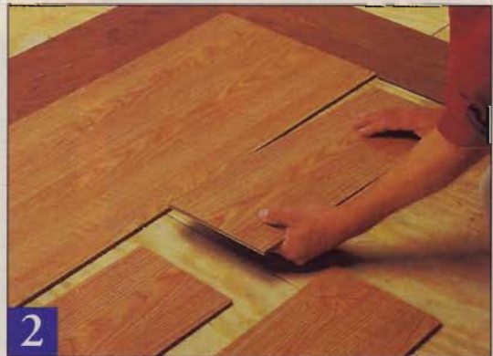
2 Establish a baseline along the longest, straightest wall. Dry-fit the planks together to check the flooring alignment and to create the proper spacing for any inset borders.
