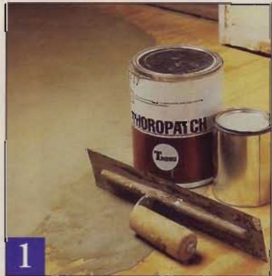
1 Use a leveling compound to fill in any depressions. Feather the edges of the compound to reduce sanding after it dries.
