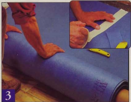
3 Roll out a width of the backing pad and cut it to length with a utility knife. Roll out additional widths, butt the edges — don't overlap them — and join them with masking tape.
