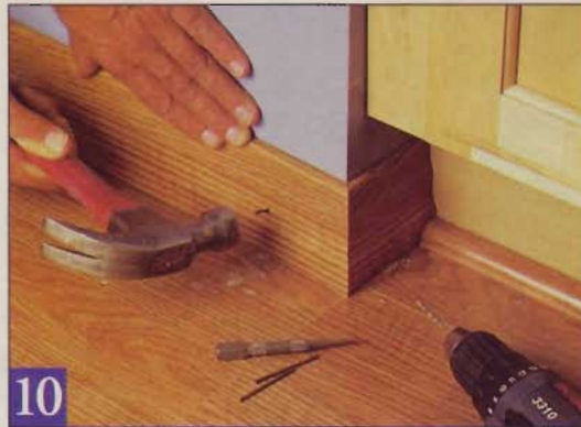
10 Drill pilot holes through the laminate-covered base molding and quarter-round before driving the finish nails. We used a nail set to sink them just below the laminate surface.
