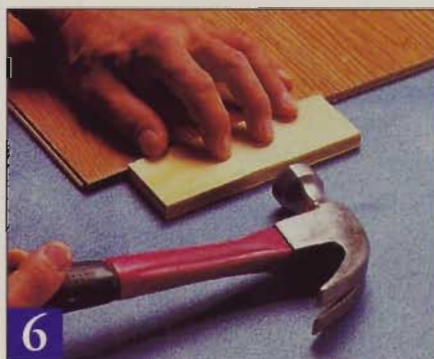
6 Tighten up the joints using a hammer and tapping block that's grooved to protect the tongue — the MDF core damages easily.
