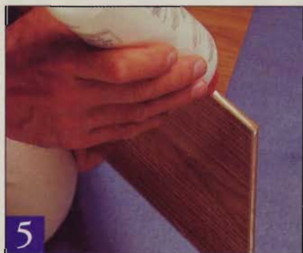
5 Apply glue only to the edge and end grooves of a plank. The glue bottle nozzle helps place the correct amount of glue in the joint.
