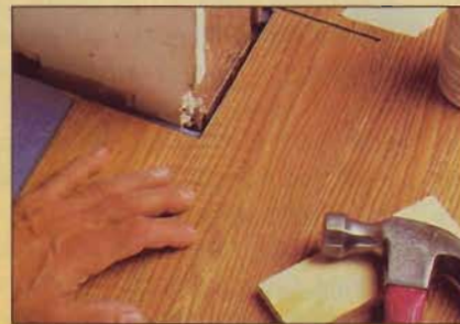
Notch an L-shaped plank to fit around the door jamb. Apply glue, slide the flooring in from the end, then tap it firmly into place.
