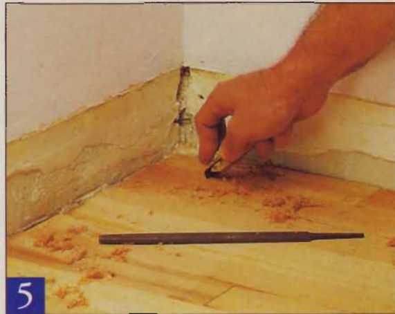
5 Use a hand scraper or a file to remove old finish in corners and hard-to-reach areas. An orbital finishing sander works great too.
