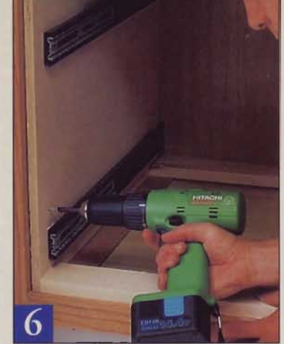
Drive two #8 x 1 1/4" screws through the box sides into each side spacer to anchor the box in the cabinet.
