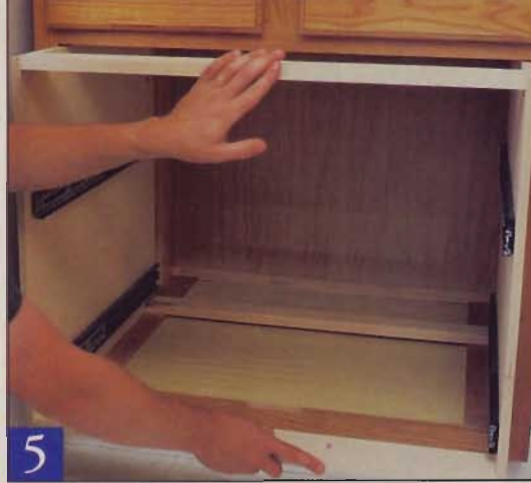
Slide the box into the cabinet — your spacers should center the box in the opening. Too much play? Try spot-gluing paper shims (playing cards are ideal) on the spacers.
