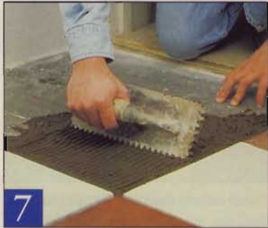
7 Spread 2-3 cups of mortar on the floor, then comb it out with the trowel's toothed-edge.
