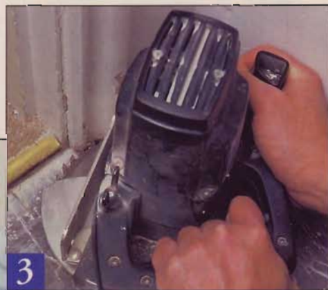
▲ Cut the bottom of the door casing so the tile can slip under. Renting a casing saw (shown) is fine, though you can easily complete this step with a fine-toothed hand saw.
