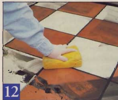
12 Clean excess grout off tile with clean water and a sponge. Change water often.
