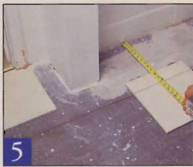
5 Align tile marks with baseline and measure for the cut tile in front of the tub.
