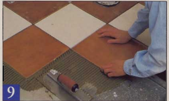
9 Lay tile in small areas, and be sure to check often that all tile remains square to the first row along the baseline.
