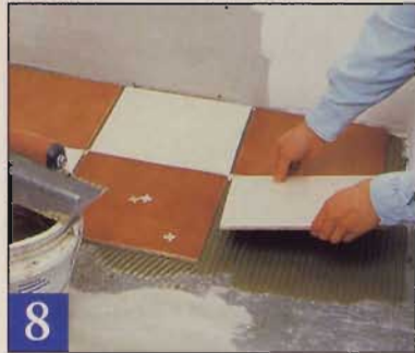
8 Begin tiling in the "square" corner. Twisting tiles a little ensures good mortar coverage.
