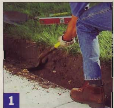
1 Dig a rough trench to establish the location of the wall. Fine-tuning will come later, when the posts are in.
