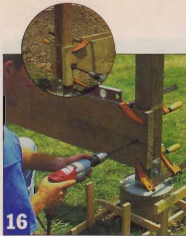
16 When the beams go up, clamps hold them until you get height and level adjustments made. Then drill and bolt.
