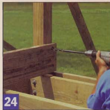
24 The front rim joist for the tier deck is bolted in place, but gets its support from the main deck joists below it.
