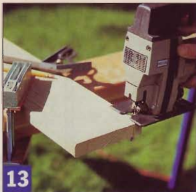
13 Use a jig saw to notch the front corners of the rail caps. This relief lets them nest snugly behind the fascias.
