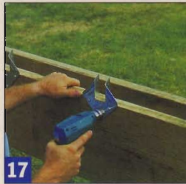
17 Transfer the joist layout marks from the ledger to the beam, then fasten a hurricane tie at each joist location.
