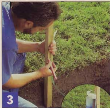
3 Drive stakes at the ends of the wall, then transfer level marks to run a string between them.
