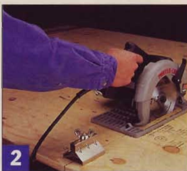
2 Once you've cut partway through the sheet, install a Kerf Keeper to help keep the stock aligned and supported.
