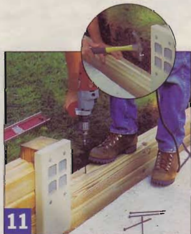
11 Nail a spline in the rail's top groove, then set the next rail in place and fasten it with several 6"-long screws.
