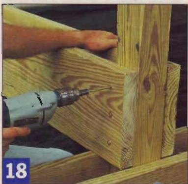
18 Install the joists at each post first, with the ends flush with the post face. I used Simpson 'SDS' lag screws here.
