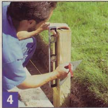
4 Set the posts temporarily in place with crushed rock underneath, then mark the height for cutting. The lower string aligns the front faces of the posts.
