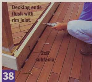
38 The diagonal decking orientation will require an extra 2x8 subfascia (with 1/2" spacers) to support the ribbons.
