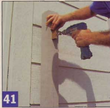
41 Mounting blocks made from ipe were fastened to the posts with heavy 3½" screws. These support the railing.
