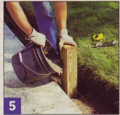
5 With the crushed rock still intact (for drainage), set each post in place and recheck the height. Then pour concrete around it and recheck plumb.
