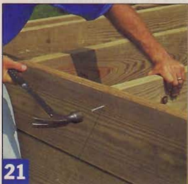
21 After bolting the rim joist to the posts, nail through it into the end of each joist. Check joist alignment as you go.
