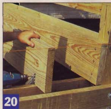
20 With a string line to keep the ends of the field joists aligned, fasten them to the hurricane ties and joist hangers.
