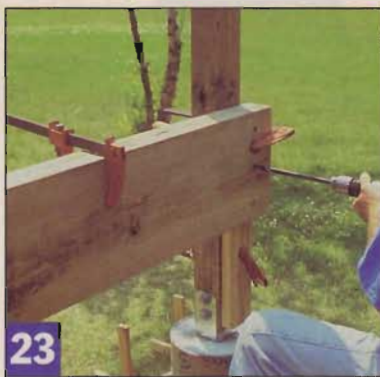
23 The double 2x12 beam for the tier deck gets bolted together inside the posts, rather than straddling them.
