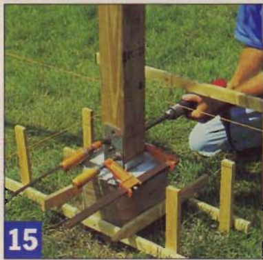
15 With the post base still clamped, drill through the bolt holes in the metal bracket and install the bolts and nuts.
