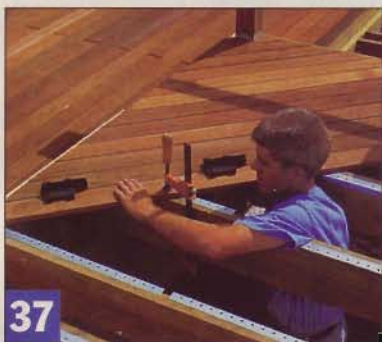
37 Orienting decking diagonally defines height changes between levels. Use clamps to keep boards from shifting.
