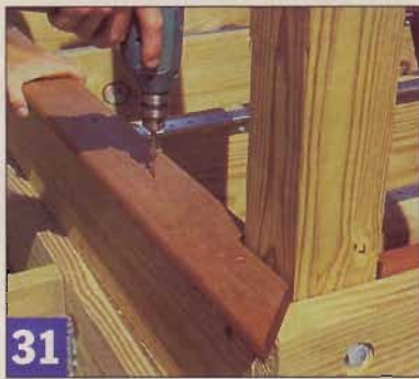
31 Unlike the “field” decking, the ribbon boards must be fastened from above with screws. Painted screws blend in.
