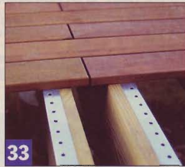
33 Splices add an interesting pattern to the deck surface. Place them over the double joists so water drains through.
