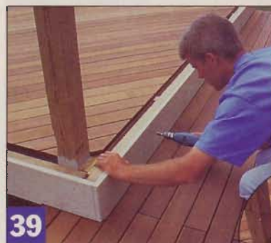
39 A 1x8 fascia, stained to match the house siding, covers the subfascia before the ribbon boards go on.
