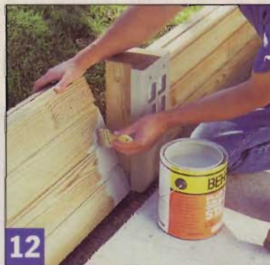
12 Apply paint or stain while you can still tilt the rail sections clear of the post fascias. I used solid-color latex stain.
