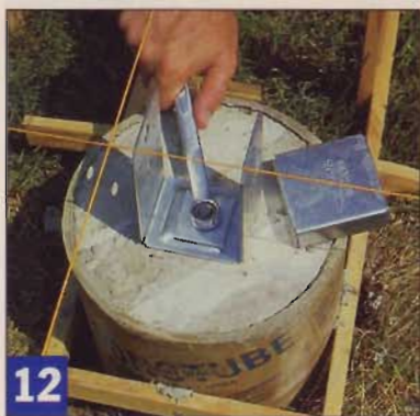
12 Realign the guide strings (to the post edges) to install the post brackets. The standoff cap covers the nut/bolt.
