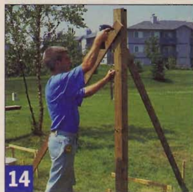
14 Tie temporary braces to wood stakes and to the top end of each post, so the post alignment is kept intact.
