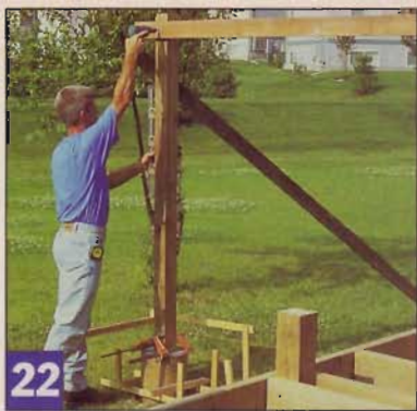
22 Like the main deck, the tier deck construction begins with bracing posts, then drilling and bolting them in.
