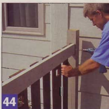
44 With the upper and lower cedar rails installed on the inside, fasten the railing assembly to the mounting blocks.
