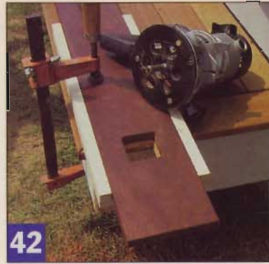
42 To add the detail to the wide balusters, I used a router jig and a flush-trim bit. Rough out with a jig saw first.
