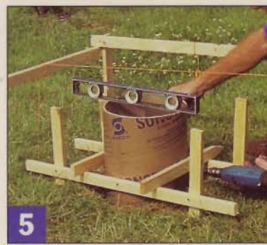
5 Rest a second pair of crossbars on the first pair, check the form for level in the other direction, then drive screws to "lock" the form where it sits.
