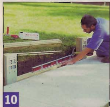
10 After laying a gravel drainage bed in the trench, set the first rail in place and tamp it until it sits perfectly level.
