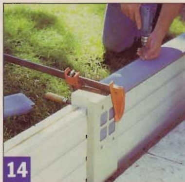
14 After routing the edges of the rail caps with a roundover bit, fasten them in place with galvanized deck screws.
