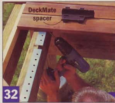
32 With a DeckMate to space the boards, the decking gets fastened from below. Note cleat used to keep ends aligned.
