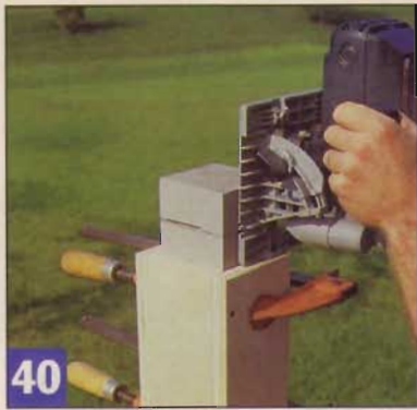
40 When it came time to cut the posts to final height, I clamped a plywood jig in place to guide and support the saw.
