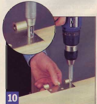
10 Using a self-centering (Vix-type) bit is the most reliable way to drill accurate pilot holes for the hinge screws. For heavy doors, use 1" or longer screws.
