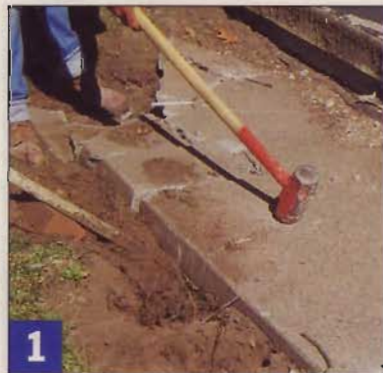
1 Nothing beats a sledgehammer for breaking up concrete. Those with uncallused hands take heed — wear gloves.
