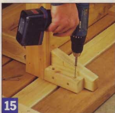
15 Drill two staggered pilot holes in the table cleats at each board location. Apply construction adhesive to each top board, then screw the cleats down.
