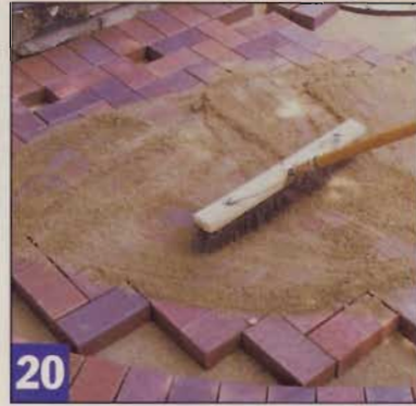
20 Spreading sand into the gaps between bricks solidifies the pattern. Avoid getting sand in the remaining holes.
