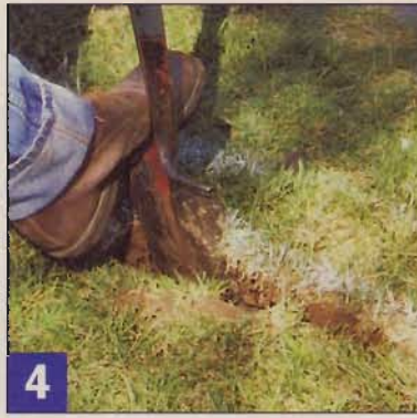
4 There's no shortage of handwork here, especially when it comes to cutting the walkway route in the sod with a spade.
