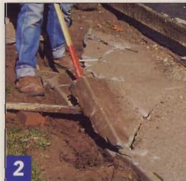
2 Pry up stubborn sections and insert a piece of concrete. A good whack with the hammer should crack the section.
