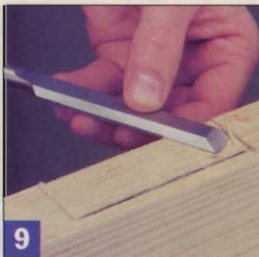
9 Freehand routing will leave some waste wood around the perimeter of the hinge mortise. Use a sharp chisel to clean up right to the edges.
