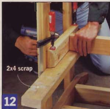
12 Clamp a piece of 2x4 scrap to the center rail at each end. Rest the lower stretchers on these "ledges" while you drill the 1/4"-dia. pilot holes.
