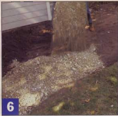
6 Properly compacted, crushed stone and dust will provide a firm foundation for the bricks. It also improves drainage.
