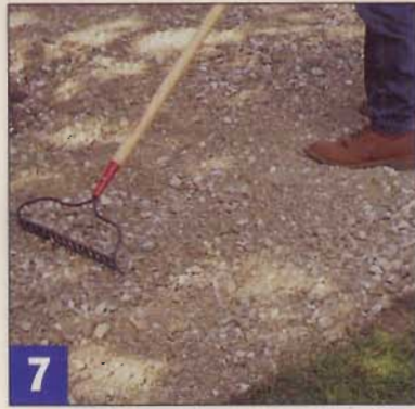
7 Rake the stone into a 3"-deep layer. Make sure the stone pathway is wide enough to support the edging.
