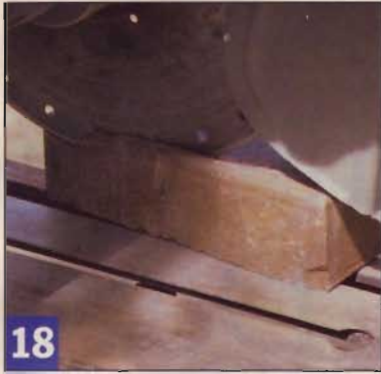
18 To follow sharp curves requires that you taper the bricks, a task easily accomplished with a brick cutting saw.
