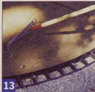
13 Rake the sand so it extends over every inch of the path. Sand provides a firm, uniformly supportive bed for the bricks.
