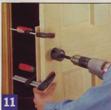
11 Carefully layout the hole centers for the lockset, and clamp scrap wood to the door to prevent tearout as the hole saw exits the workpiece.
