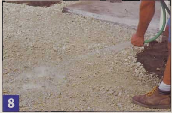
8 Compacting the foundation is critical to the long-term success of your walkway. It starts with watering the stone.
