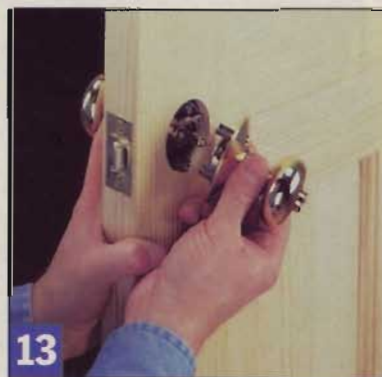
13 With the latch faceplate nesting flush with the door edge, the tail of the assembly will align with the lockset cylinder. Screws secure the handles.
