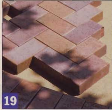
19 Once you lay the first few tiers of the herringbone pattern, the bricking sequence is easy to repeat.
