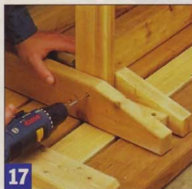
17 Position the outer rail, clamp it to the leg, and drill pilot holes. Unclamp the outer rail, then glue and screw it in place with #8 x 4" screws.
