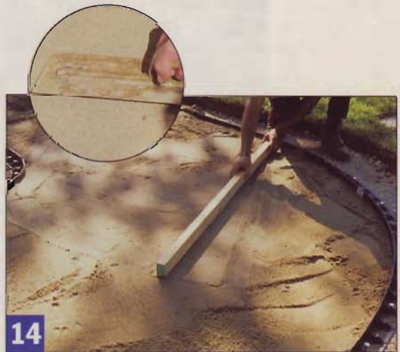
14 Work the sand to a uniform depth and keep it flat using a straight-edged 2x4. A trowel is handy for smaller areas.
