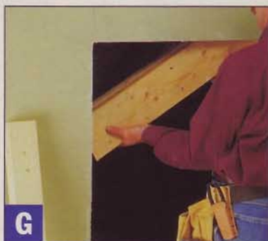
G Swing the header — a pair of 2x6's with 1/2"-thick plywood in between — into place on top of the trimmer. Then install the other trimmer.
