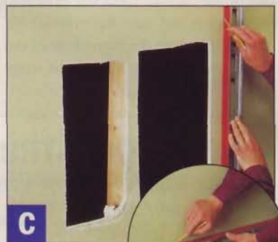
C Use a level to mark the sides of the carcass hole plumb, and the top and bottom level.
