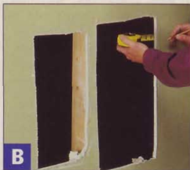
B Measure from existing studs to mark the edge of the hole for the carcass. Leave the drywall 1 1/2" proud of the studs on both sides of the hole.
