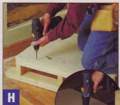
H Assemble the dresser platform, lift it into the wall cavity, then secure it to the front sill plate.
