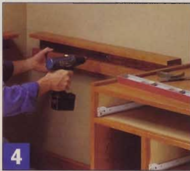
4 Position the wall cleats along the level lines and drill mounting screw holes at the stud locations. Drive #8 x 2" screws to hold the cleats in place.
