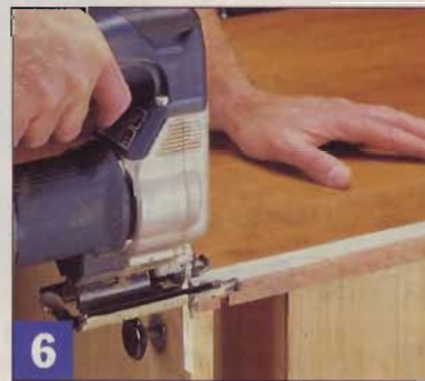
6 Use a jig saw equipped with a fine-toothed blade to trim each pedestal along the scribe line. Use a file to make fine adjustments to the fit.
