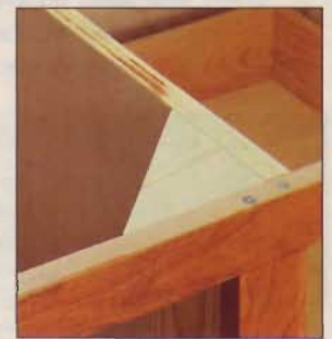
A single stile and a ¾"-thick plywood divider panel separate compartments in the large base unit.
