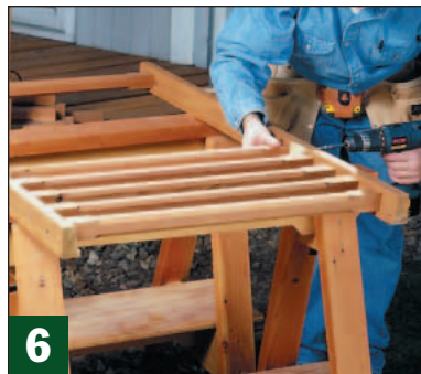
6 Starting at one end, use a spacer to position the balusters. Then attach them to the stringers with 3" screws.
