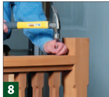
8 Center the stringers on the width of the rails. Drive 6d galvanized finish nails to hold the sections in place.
