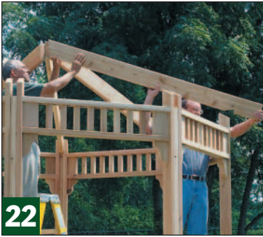
Attach two hip rafters (U) to the king post (T) and lift the assembly into position. Check the fit at both ends.
