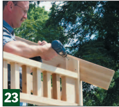
After making any adjustments to the rafters, secure them to the posts by driving screws in from both sides.
