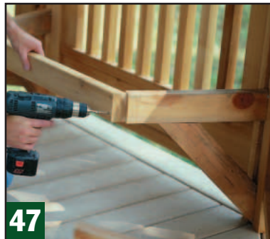
47 Bevel the stretcher ends at 22 \frac{1}{2} ° so the stretchers reach from center to center on the supports. Screw them in place.
