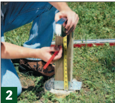
2 Now set a post in the connector on the high footing, mark the height of the floor joists, and cut the post to length.
