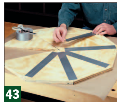
43 Tape the triangles edge-to-edge with the bevels down. (That extra space will close up when you "raise" the roof.)
