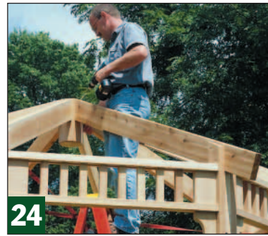
Install the remaining hip rafters in opposing pairs. Use a ratcheting tie-down strap to pull the walls into place.
