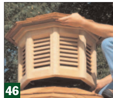
46 Measure and mark 12" down from the center of the king post along each hip. Use these marks to center the cupola.
