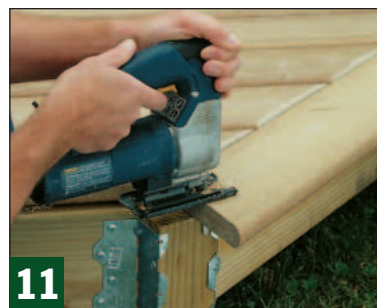
11 To create an opening in the border planks for a metal strap, use a jig saw to cut a slot that's flush with the post.
