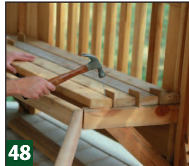
48 Miter the slat ends to meet the centerline of the supports. Use spacers to hold them while you nail the slats down.
