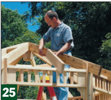
With a stub rafter set at right angles to the wall, mark its location on the hip rafters on both sides.
