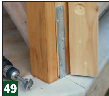
49 Position the fascia (MM) on the post and hit the board with your hand. Drill a counterbore at the screwhead dimples.
