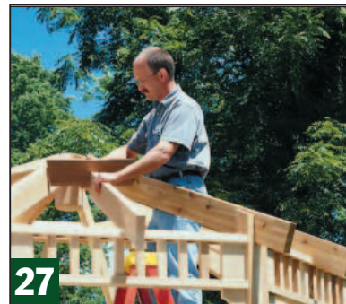
Trim a compound angle on the ends of the header (W) until it fits between the hip rafters and against the stub rafter.
