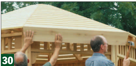
Hold a 1x8 fascia (Z) against the rafters and mark the compound angle needed. Fit each board to the previous one.
