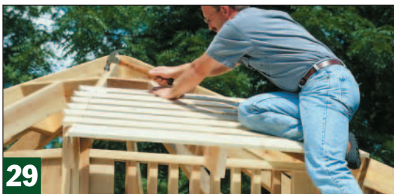
Tack 1x4 roof slats (Y) in place, leaving them extra long on each end. Use a chalkline to mark them to length.
