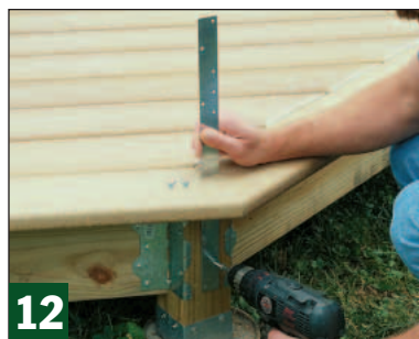
12 After slipping a 18"-long "tie-down" strap through the slot, fasten it to the outer face of the post with screws.
