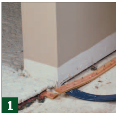
1 To prepare the subfloor, I started by using a wrecking bar to pry off the tack strips that held the carpet.
