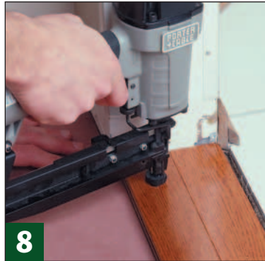
To create an attractive transition between rooms, I face-nailed a double row of trim strips in the entryway.
