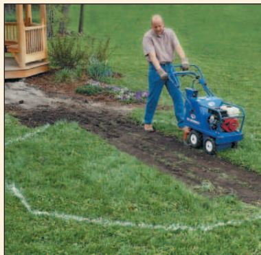
After spray painting the outline of the walkway, a gas-powered sod cutter makes quick work of removing the sod.
