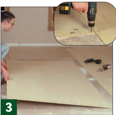
To "raise" the height of the wood floor, I screwed sheets of \frac{1}{4} " plywood perpendicular to the subfloor.
