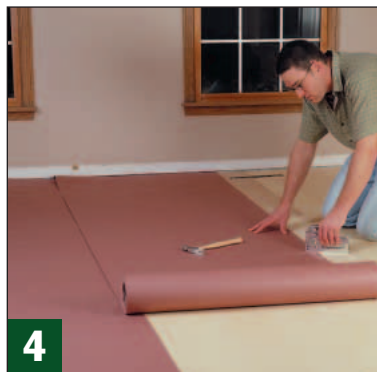
Next, to create a moisture barrier, roll out construction paper in overlapping strips and staple it in place.
