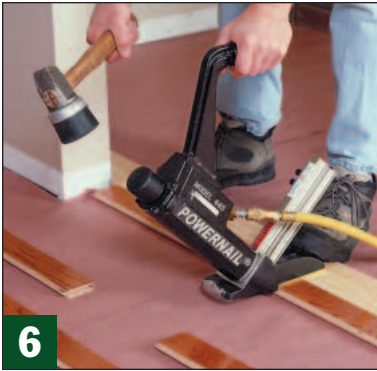
6 After screwing a wood cleat to the subfloor, set the first flooring strip against it and nail it in place.
