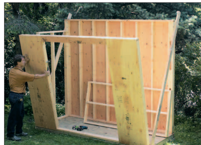
A couple of diagonal braces hold the back wall plumb as you set the end and front walls into position. The walls are fastened to the floor and to each other with 3" deck screws.
