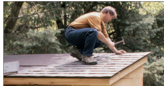
Staggering the seams in between courses is part of making a roof watertight. Run a staggered pattern of shingles to the peak before shingling the length of the roof.
