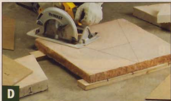
D Use a separate template to lay out each wedge-shaped hearthstone. Then cut the stones to shape with a circular saw and diamond blade.
