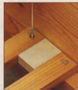
▲ A 1 1/2"-wide scrap block creates consistent spacing when installing the bottom slats.
