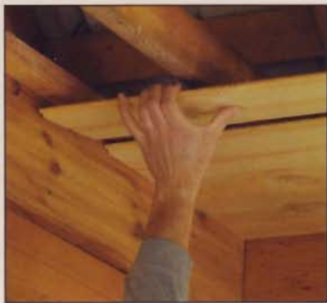
▲ Pine car siding with pre-cut tongue-and-groove joints conceals the trusses and creates an attractive ceiling.
