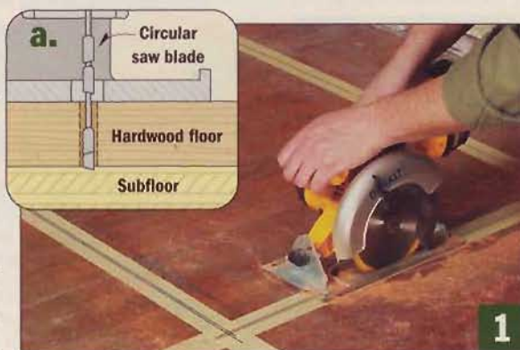
▲ To cut the opening for the hearth, I used a circular saw with a special nail-cutting blade. Masking tape makes it easy to see layout lines.
