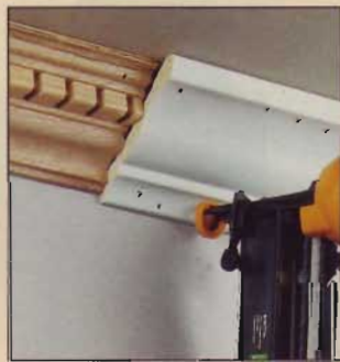
▲ NOSE PAD CLEARANCE This test showed us whether there was any interference when nailing into the contours of crown molding.
