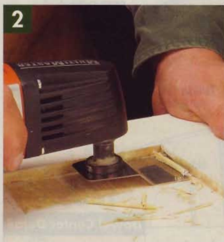
▲ A stiff scraper blade makes easy work of removing multiple layers of paint. The same blade removed vinyl, carpet, and carpet padding effortlessly.
