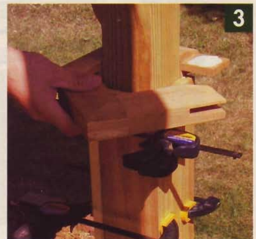
▲ To install the mid-cap, remove the screws to separate it into the two L-shaped sections again. Then apply exterior glue, fit the sections together, and clamp the joints.
