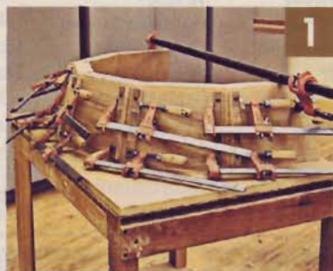
▲ To make a curved molding, Lynn starts by gluing pieces together into a trapezoid, using splines for alignment.
