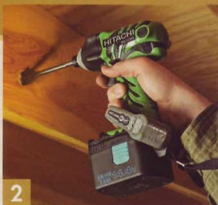
▲ When drilling holes through floor joists to run wiring, the compact size of the impact driver makes it a natural.
