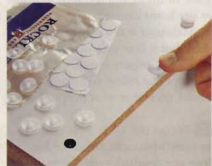
Exposed holes can be covered with either plastic caps that lock into the screw heads or self-adhesive "stickers."
