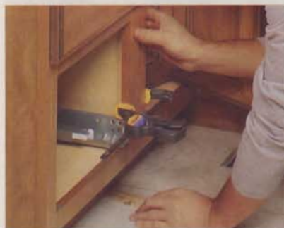
5] Shim the cabinets to level them and align them with the level line on the wall. Also be sure to align the face frames.
