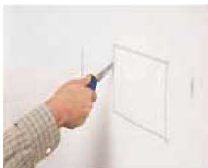
2] Using a drywall saw, cut an opening between the studs, so you can make sure there are no pipes or wires in the way.
