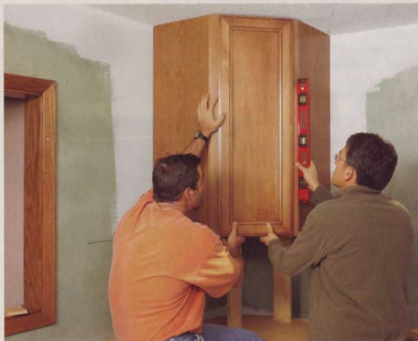
10] Enlist a helper and use "kicker" boards to help support heavy upper cabinets. A corner cabinet like this may require shimming on both walls to true it up.
