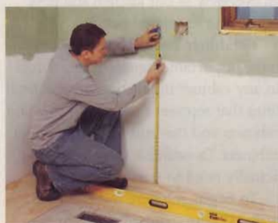
1] Locate the high point on the floor. Transfer that elevation to the wall, and then measure up 34½".
