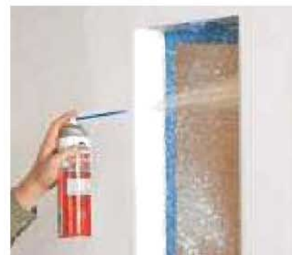
8] If the wall around the niche is textured, you can easily match that look by using a can of spray texture.
