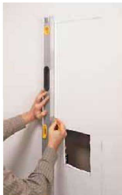
3] After measuring and marking the top, bottom, and sides of the opening, lay them out using a 4-ft. level and pencil.
