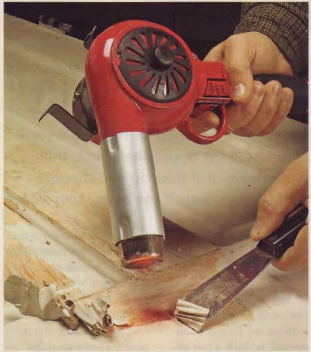
A heat gun quickly softens multiple layers of paint, allowing them to peel up easily in large strips. Just be sure to wear a respirator when removing paint that may contain lead.
