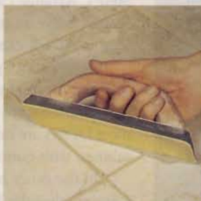
9] Use a sponge float to level the grout and ensure all of the joints are completely filled.
