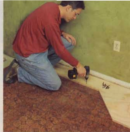
2] With careful measurement and cutting, we built platforms for the new cabinets.
