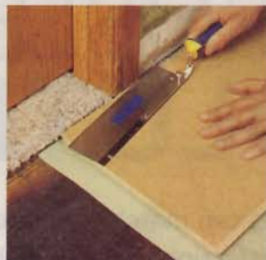
4] Use a tile panel as a guide as you cut door jambs, so the tile can fit underneath.
