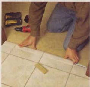
7] Install transitions in the doorways. Use the ones provided, or make your own.
