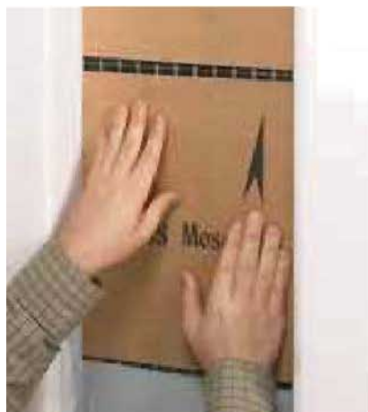
3] Align the sheets of tile in the opening, with an equal space between each sheet, and press them into place.
