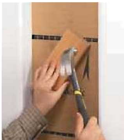
4] Using a hammer and a scrap block, lightly tap the surface of the tiles to seat them securely in the mortar.
