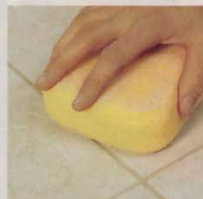
10] Clean up excess grout with a damp sponge and special wipes from Edge Flooring.
