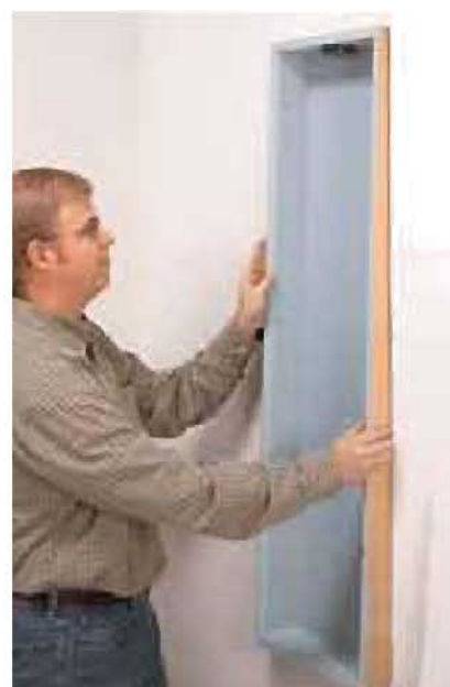
6] Slide the box into position to check the fit, and make any needed adjustments before screwing it in place.
