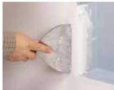
2] After mudding over the tape, smooth it over the rounded corners using a 6" putty knife.
