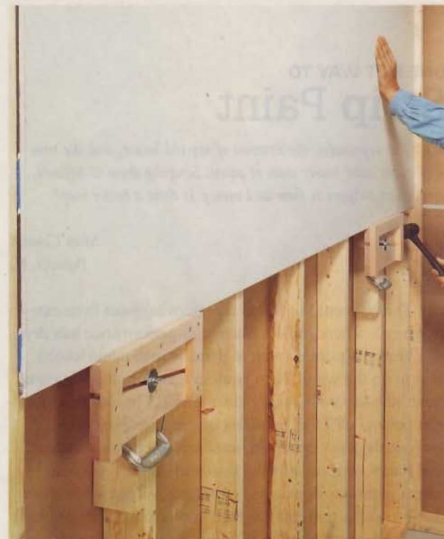
Clamping two "lifts" to the wall studs makes it easy to support a sheet of drywall. Tap the lifts sideways to raise the sheet to the ceiling, freeing your hands to drive screws.
