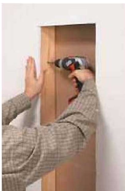
5] Frame the sides of the opening with 2x4s. You may need to add blocking to get the frame flush with the opening.
