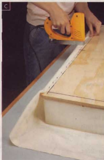
Line up the edge of the muslin with the pencil line on the base, and starting in the center, staple the material in place.
