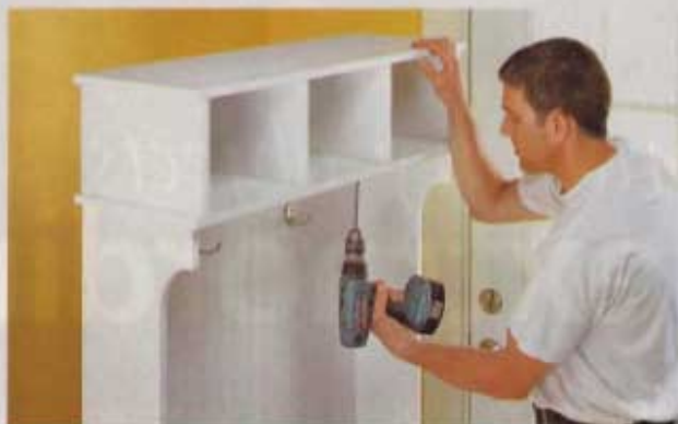
4] To secure the cubbies, drive connecting screws through the holes in the locker top and into the cubby dividers. Then drive pocket screws in through the back panel.
