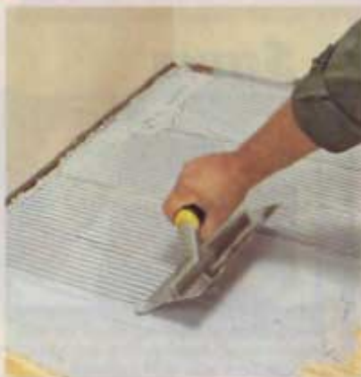
1] Apply a bed of latex-modified thinset mortar directly to the substrate using a \frac{1}{4} " x \frac{1}{4} " notched trowel.
