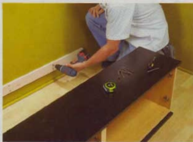
A cleat that's mounted to the wall and screwed to the studs helps support the weight of the media center and TV.
