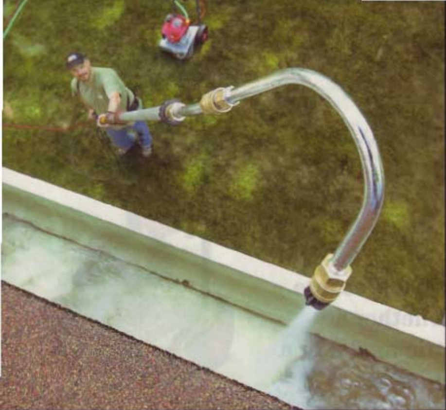
A telescoping pole, a U-shaped gutter attachment, and a low-pressure nozzle make quick, safe work out of cleaning the gutters.
