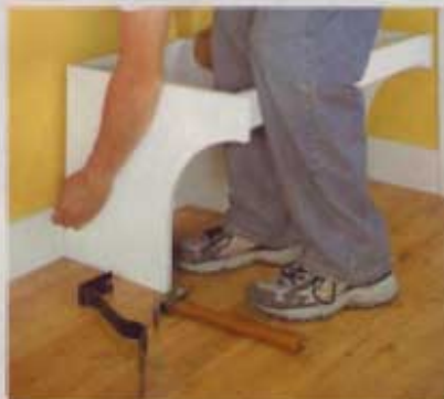
1] Set the base in place and mark the baseboard. Then cut out the baseboard, so the locker can fit tight to the wall.
