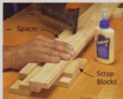
Assemble the fascia upside down, using a spacer to create the reveals and scrap blocks to steady the assembly.
