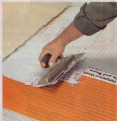
4] Use the flat edge of your notched trowel to apply a "scratch" coat of unmodified mortar to fill the cavities.
