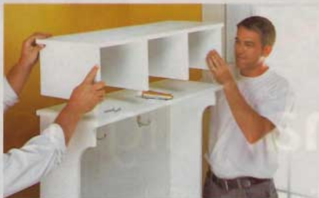
3] Add the overhead cubbies next. Apply a bead of construction adhesive to the bottom edge of the cubby ends, and then set the cubbies in position.
