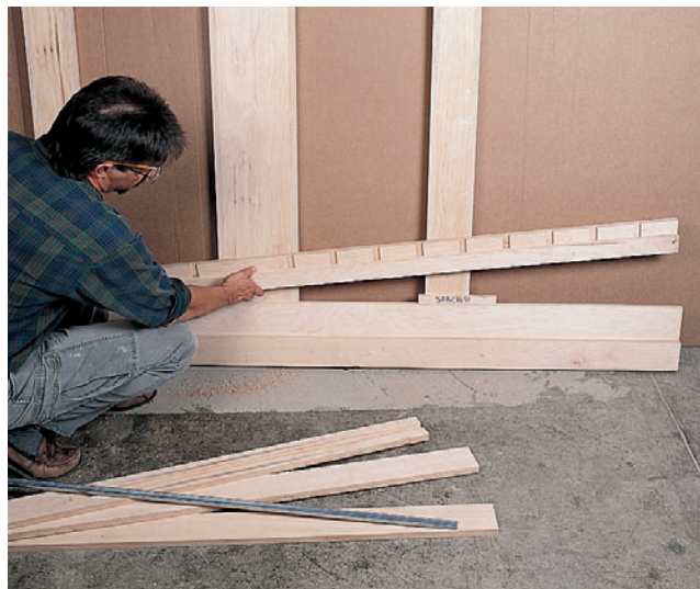
Figure 2: Spacers are an absolute necessity when aligning the horizontal members on a frame this large. To ensure accuracy, be sure your spacers are true along their full length.
