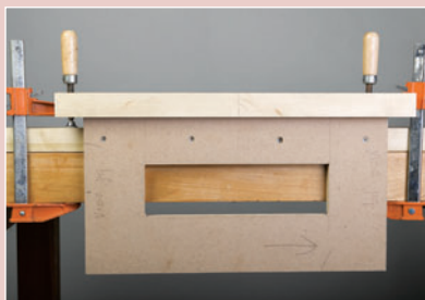
Begin the vise installation by clamping the pattern jig for routing the vise mortise in place to the benchtop.
