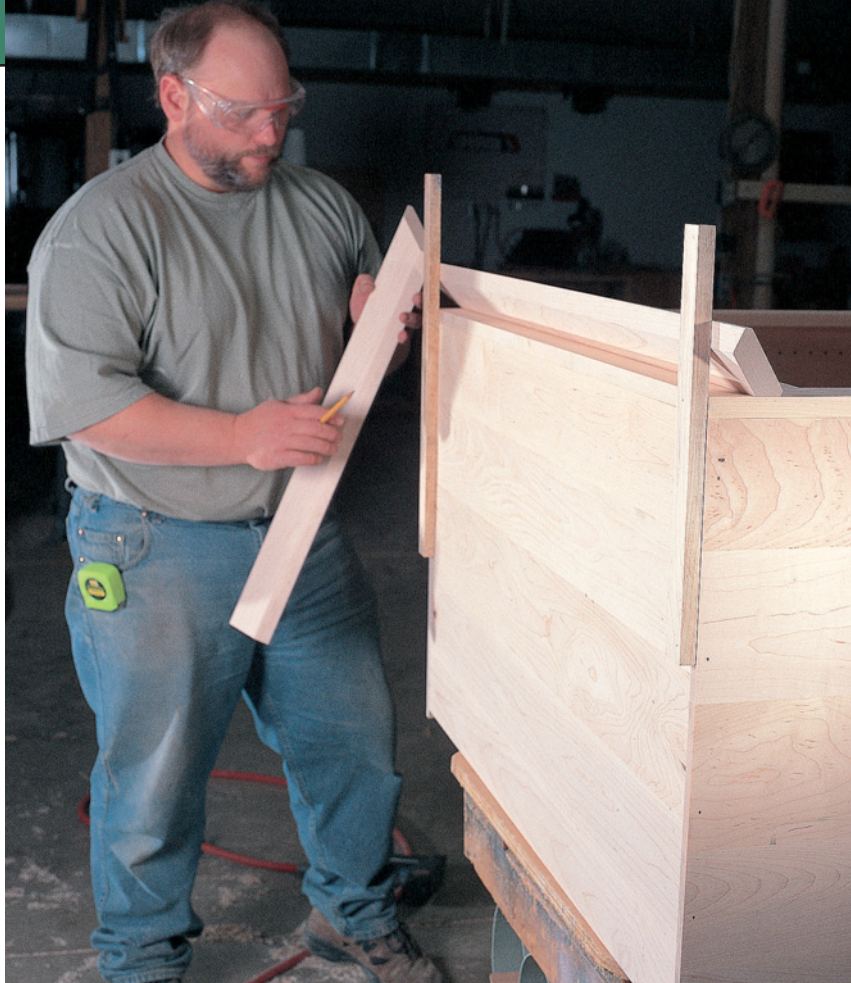
To make sure the crown moulding is flush to the top of the cabinet, I temporarily screw two scrap strips to the top of the cabinet while I align the front piece. When the front piece is attached, it's fairly easy to carry the height orientation around to the sides. Then simply remove the strips.
