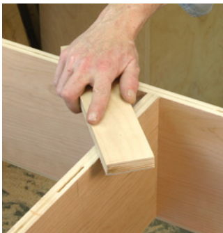
Before attaching the face frame, sand the front edges flush with a flat sanding block. I used a cloth-backed sanding belt glued to plywood.
