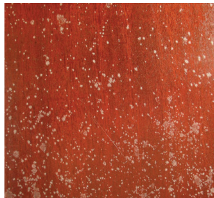
Mildew spores can be killed (to stop further growth) by washing the surface with half-and-half household bleach and water. Dry the surface quickly so the water doesn't damage the finish.
